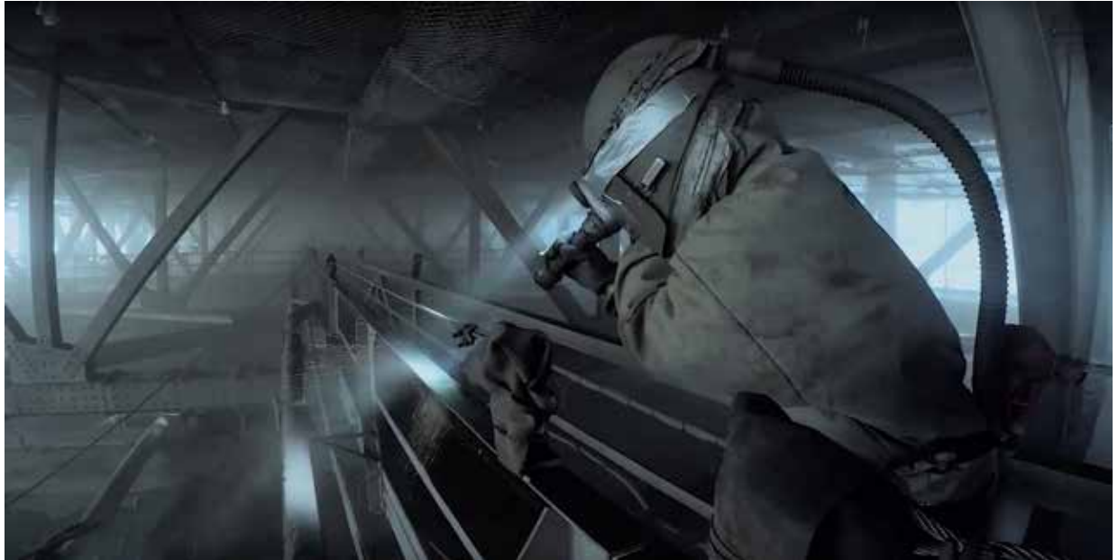
Although this photo was taken from a competitor, Bridge Bros., it gives a feel for working inside the tented area
